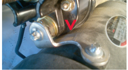
Properly installed motor strap
