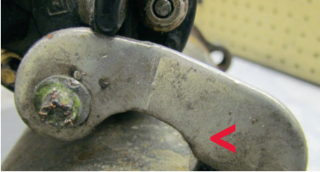
Improperly installed motor strap
